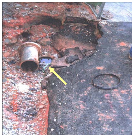
A view of a 16-inch water main that burst due to improper construction and operations.
